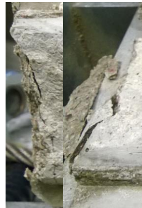
Figure 15. Closeup of the damaged front of pilot #3
