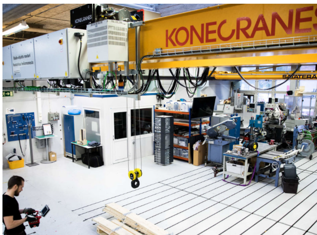
Figure 1. The smart overhead crane at the Aalto Industrial Internet Campus.
