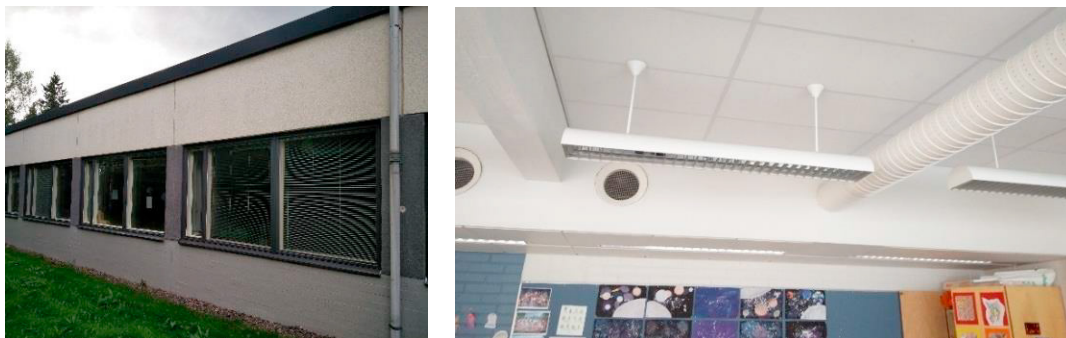
Fig. 1. (a) Studied building part; (b) A typical supply air duct diffuser and an extract air grille in a classroom.
