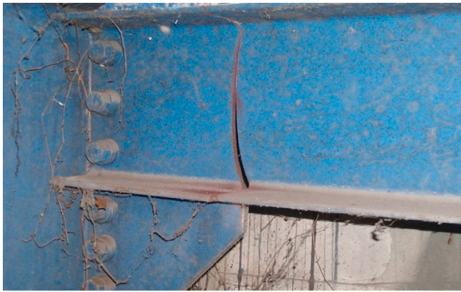
Fig. 11. Photo of a damaged cross beam of a bridge [30].
