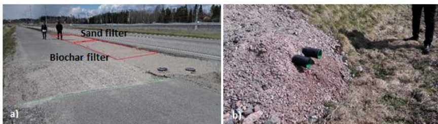
Figure A1. a) Upper part of the filters, highlighted in red. The manholes in front are connected to underdrains that convey water under the walkway to the left. b) Two drain outlets from the sand filter (left) and biochar filter (right) discharging into the ditch next to the road. (Images by Eero Assmuth)
