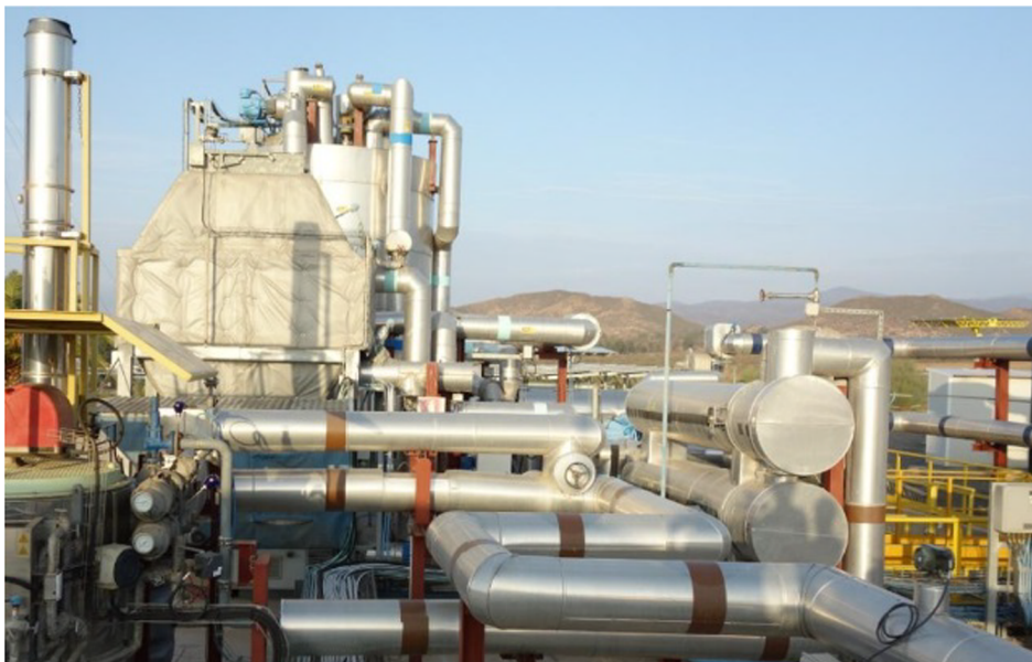
Fig. 1. A view of the MOSA facility at PSA/CIEMAT in southern Spain, showing the boiler (left, with chimney), hot salt tank with entering pipelines, a pair of heat exchangers, and insulated thermal oil and MS pipelines. The yellow safety rail on the far right indicates the pit of the cold salt tank. (For interpretation of the references to color in this figure legend, the reader is referred to the web version of this article.)
