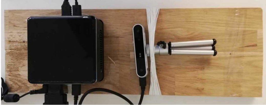
Figure 12: The mini-PC and camera installed in the factory
