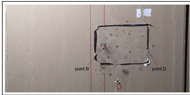
Figure 8. Mold growth was observed on the interior face of the EGS after the MCONI test. The wood frame was located between the vertical lines, the inlet pipe was located opposite the spot marked with the letter “X,” and the outlet hole was located next to the letter “O.” The black ethylene propylene diene monomer (EPDM) sealant is visible at the edges of the EGS piece, whose outer surface was additionally taped. The EGS piece was removed at the end of Phase 3 for probe installations. The board was kept intact before that point.
